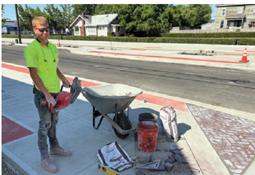
Kurt Marttila of TMC Contractors working on the brickwork at Jefferson Street and West 12th
